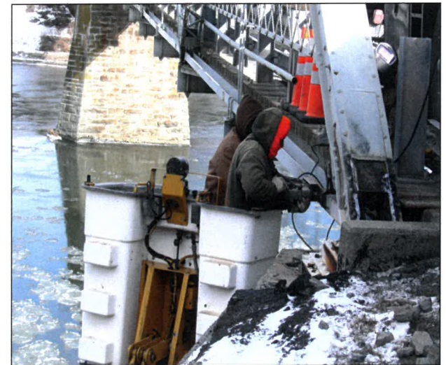
Workmen at the bridge in January 2010. Despite frigid conditions they soon finished the job. Note ice on the Delaware River.
