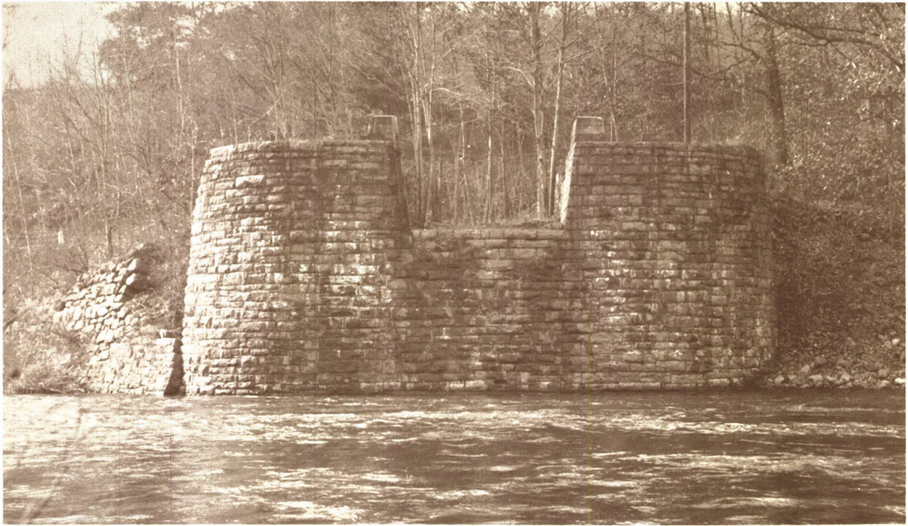
FIGURE 34.—Remains of the Lackawaxen Aqueduct. Only the west abutment survives, the east abutment and the midriver pier having been entirely demolished for the conveniently located supply of cut stone. (Historic American Engineering Record and the Smithsonian Institution.)
